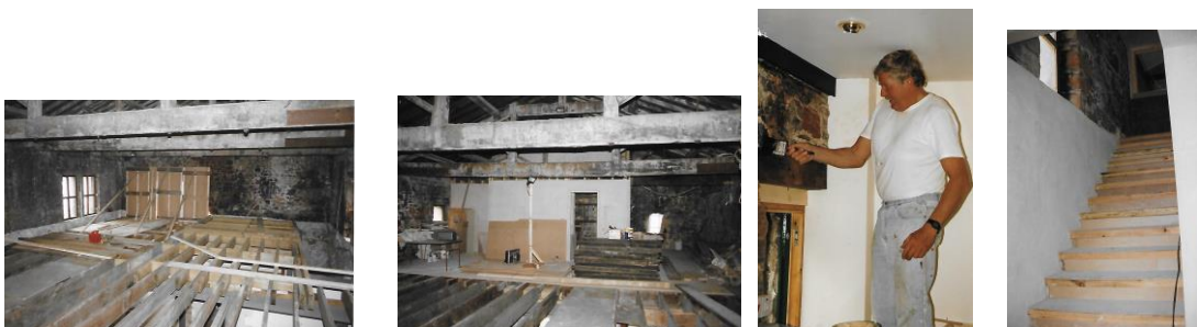
Work now started on completing the upper floors of the Tower to create the fabulous Club Room we use today.
