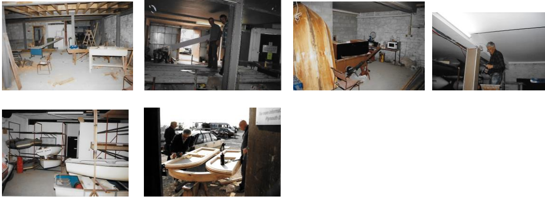
After a huge amount of hard graft by a dedicated band of members the ground floor was completed
